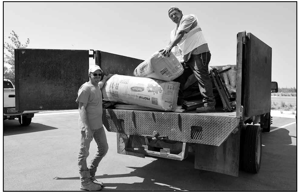
Express Interiors, Inc. of Austin is completing work for First American Title Builders in Cedar Park. L-R: Alan Woodard , superintendent for general contractor D.H. Allen , and Charlie Ontiveros take a break from gathering supplies. — ke
