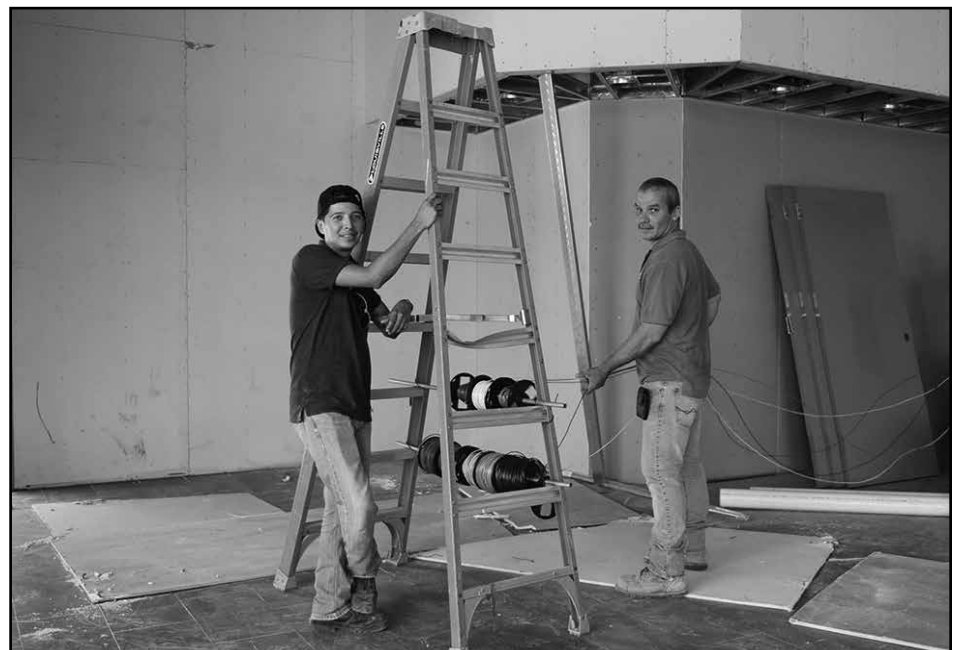
L-R: Mario Lujan and Carmelo Perez with Kumar Electrical, Inc. of Austin work on wiring for a convenience store project at 3980 Hero Way in Cedar Park. — ke
