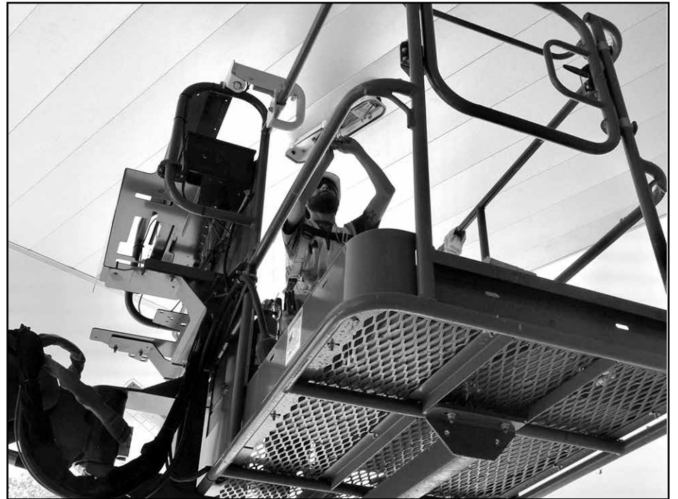
Justin Garcia with Efficient Air Conditioning and Electrical in Austin installs outdoor lighting at Lakeline Self-Storage in Austin. ARCO Murray is the general contractor. — ke
